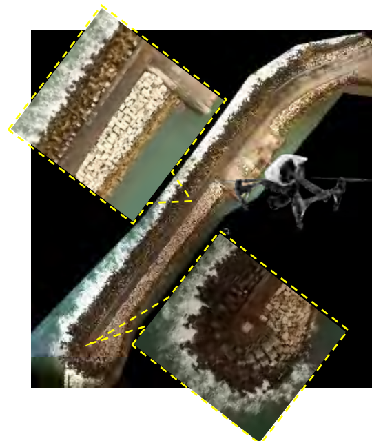
Fig. 2. Orthophoto of Ericeira's breakwater, obtained after a drone campaign, on April 24, 2018, with details of the areas of the trunk and head, at the indicated points, at a height of 60 m.
