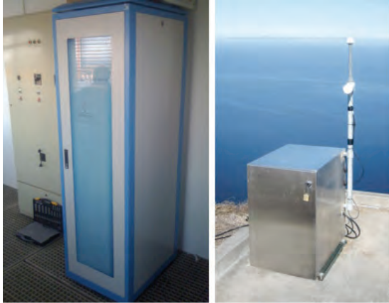
Fig. 1. Typical electronics rack solutions, standard and compact
