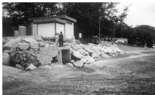
Figure 2. Aspects of infrastructures damages in Hac-Sá beach (June 2002).
